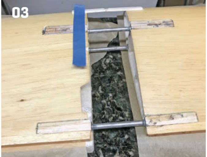
The author used cradles to align the wing panels and temporary braces to hold them in place while the epoxy dried.
